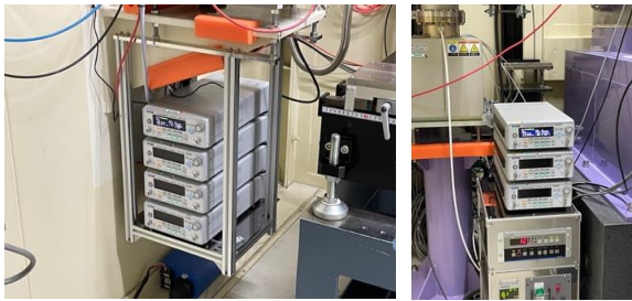
Fig. 1. Current amplifiers installed in EH1 (left) and EH3 (right). The amplifiers can be controlled via a beamline network.
